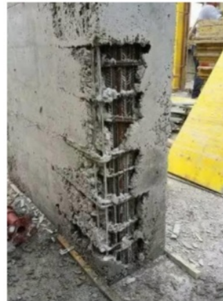
b. Poor compaction at shear wall
