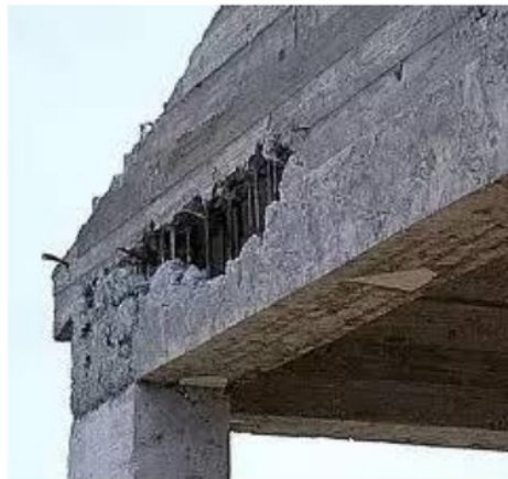
a . Poor compaction at beam-column joint
